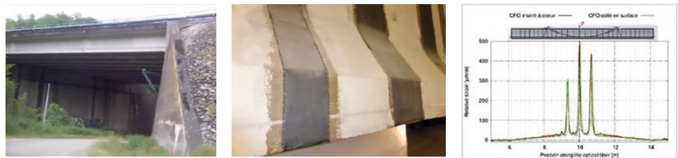
From left to right Varèze bridge, bonded fibres, deformation amplitudes as measured along the fibre and showing the location of cracks
