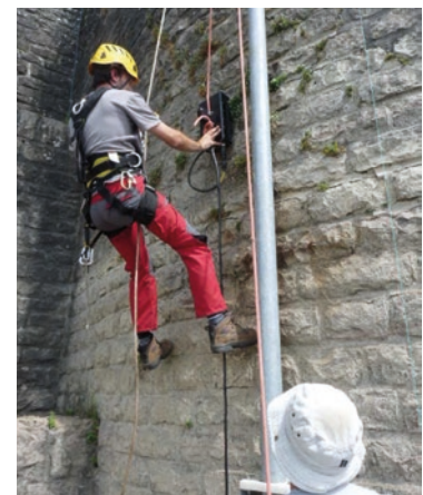
Radar measurements made by rope access technicians at the water intake tower of the Chazilly dam
