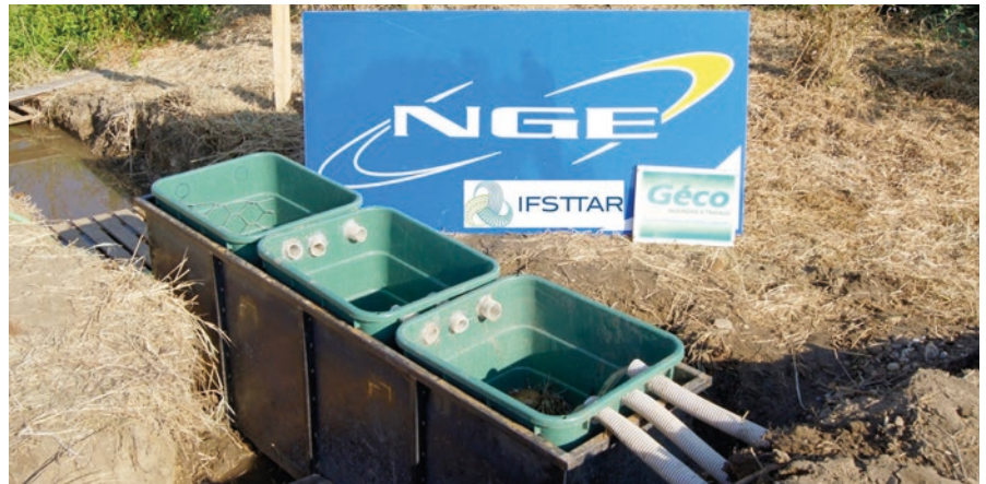
Gravitational filtration device for run-off waters
